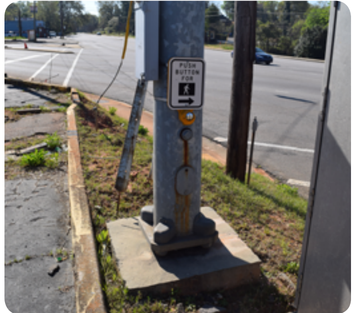
A pedestrian push button placed at the crest of a berm, in front of a utility box, and where sidewalks are lacking prevent pedestrians from being able to use this facility that aids in a safe crossing. This is at the skewed intersection of Clement Drive, River Drive, and Route 16.
