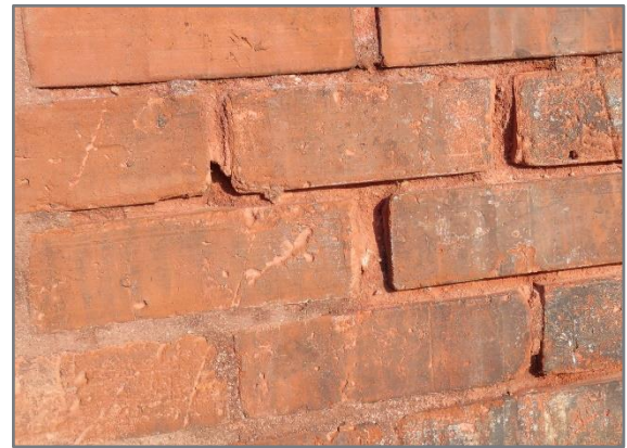
Although highly deteriorated today, the historic mortar was originally colored to match the brick
