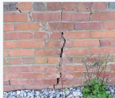
Cracks should be monitored to ensure that they are not caused by ongoing movement of the building. Active movement and expanding cracks should be evaluated by a structural engineer.
