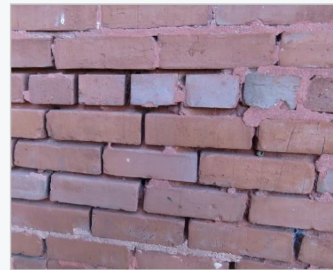
Over time, the mortar on this building has washed away almost entirely. On the right side of the photo, a poor repair is visible. Not only is the color incorrect, the mortar is too hard and has caused the brick to crack.
