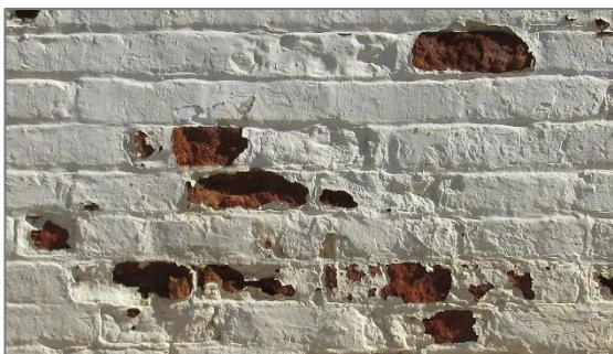
Trapped moisture in this brick has caused spalling of the brick to the point where many of the bricks have turned to dust behind the paint. More brick deterioration may be unseen behind the intact paint.
