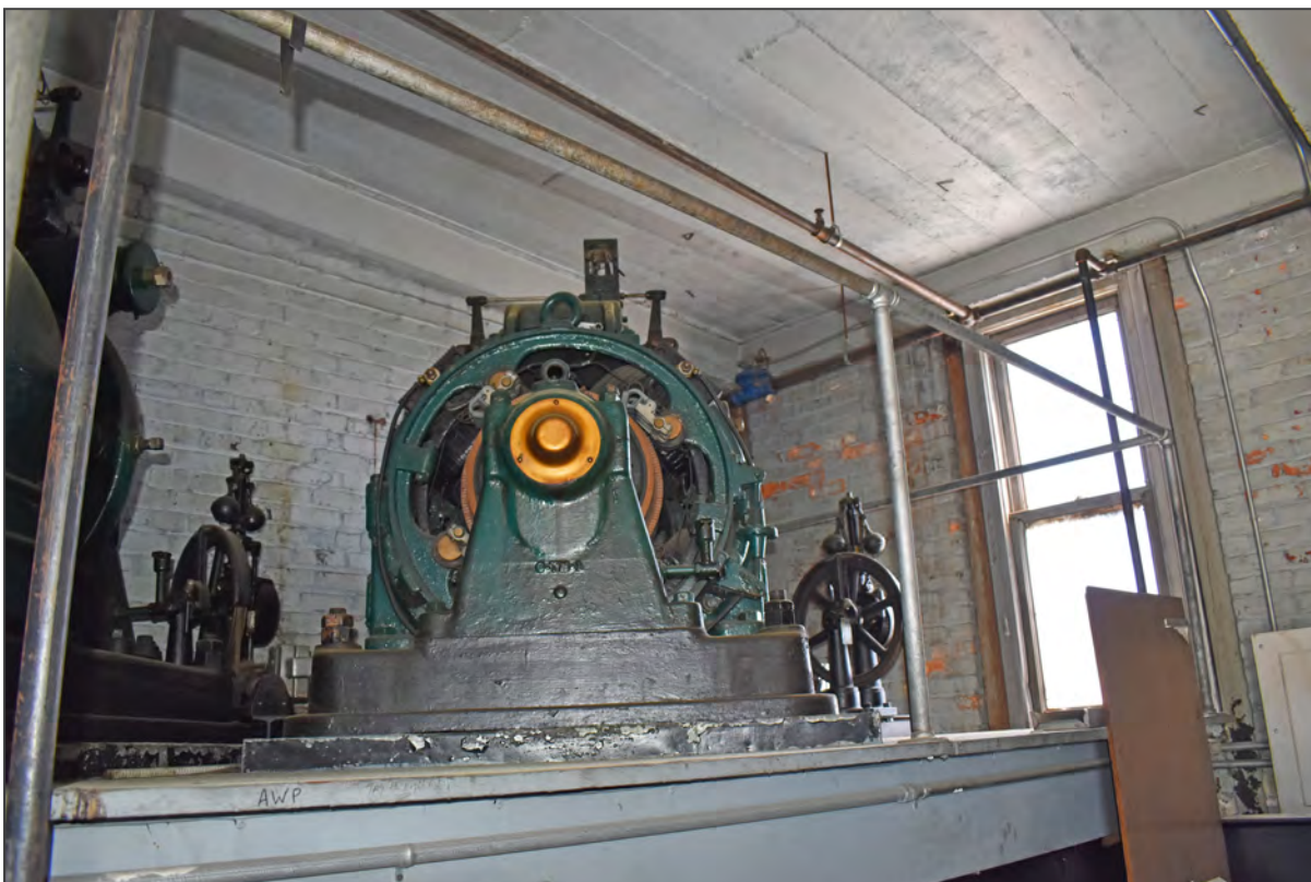
112. Roof, elevator mechanical room
