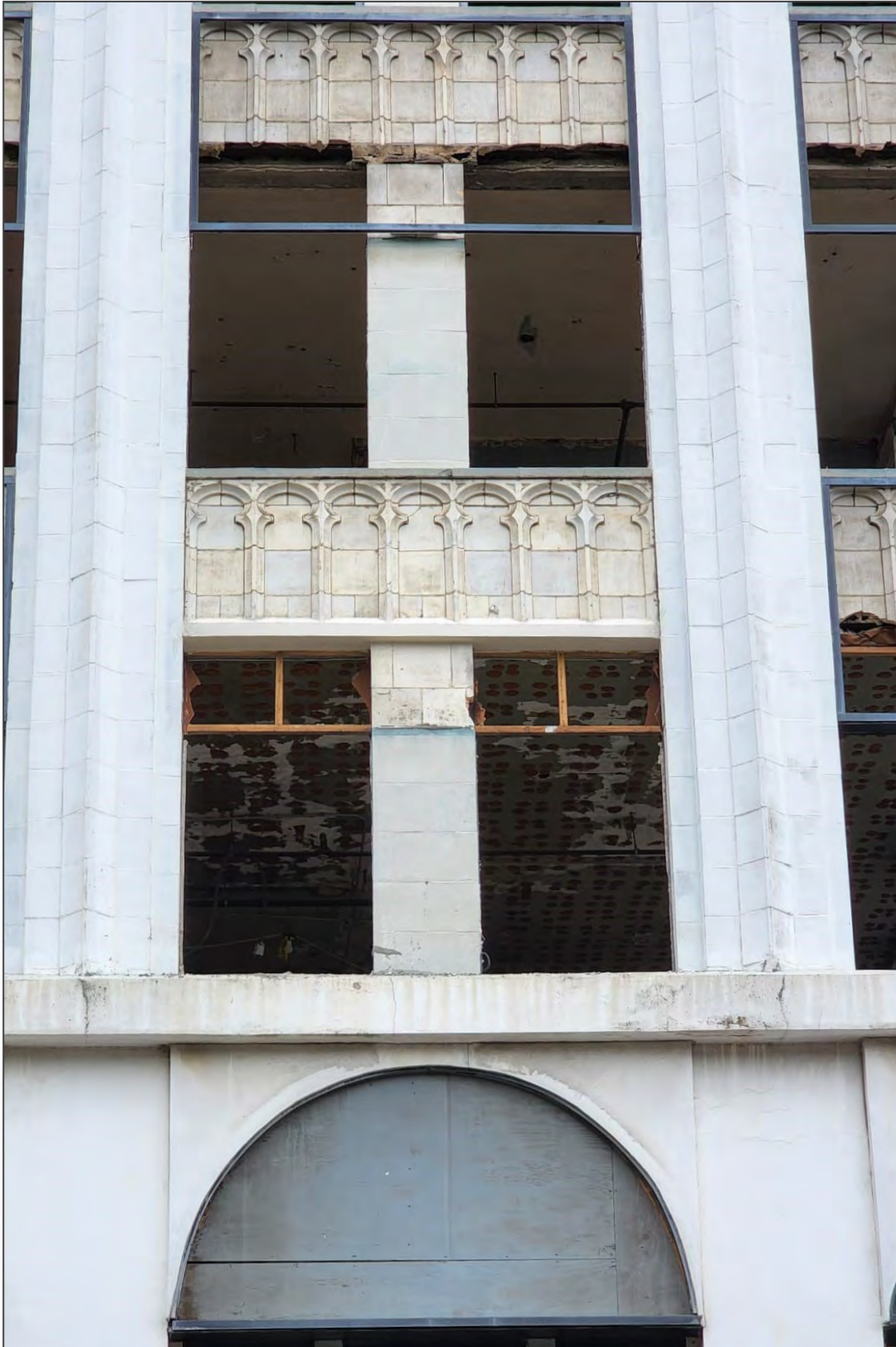
115. Example of replacement window header. Decorative tiles are original, header at the bottom is replacement painted to match.
