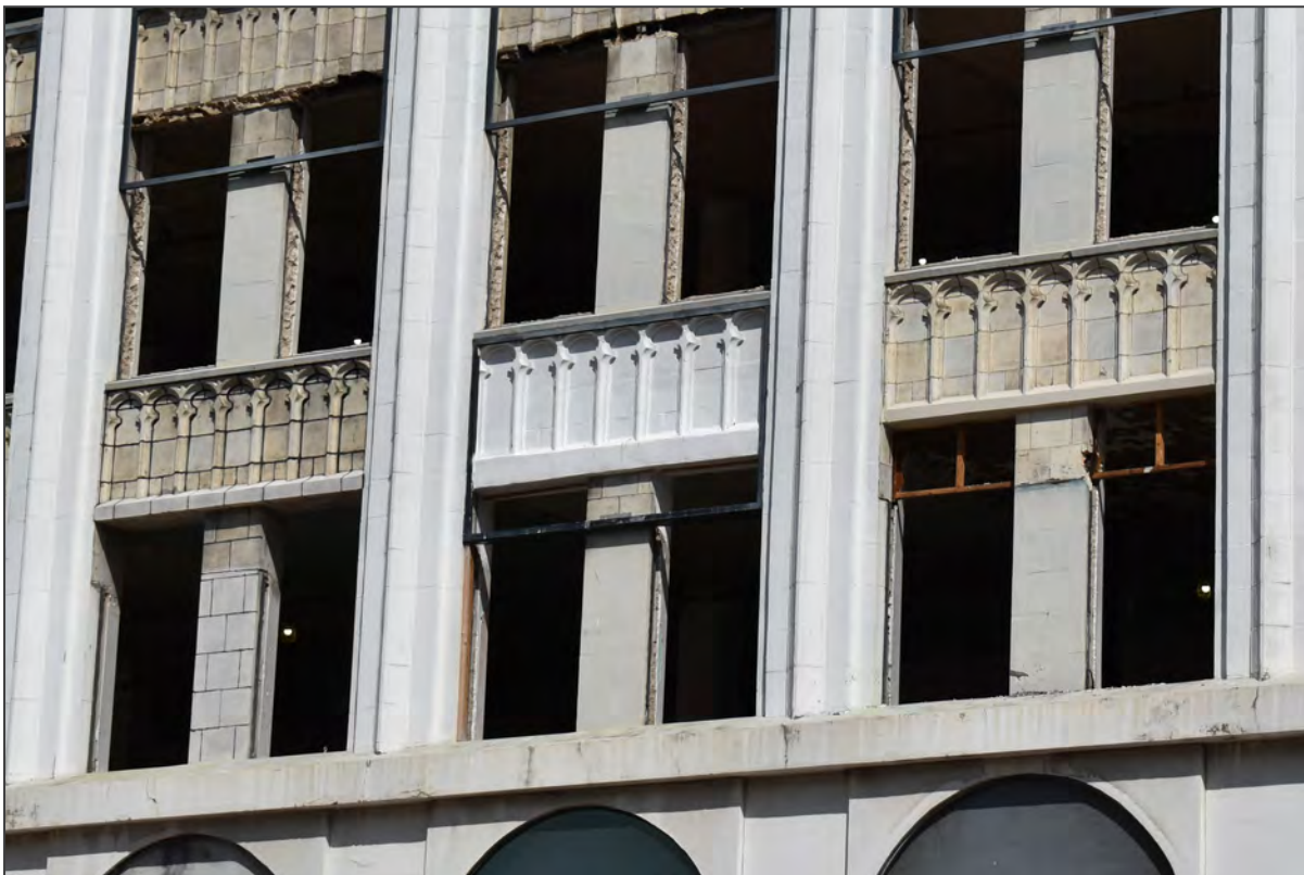
119. Uncovered terra cotta tile with replacement header (right) with replacement terra cotta panel and early header prototype (center and left).
