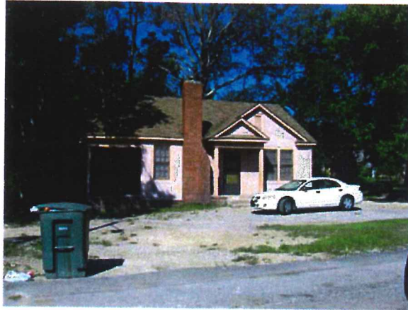
Deteriorating home in Belmont
