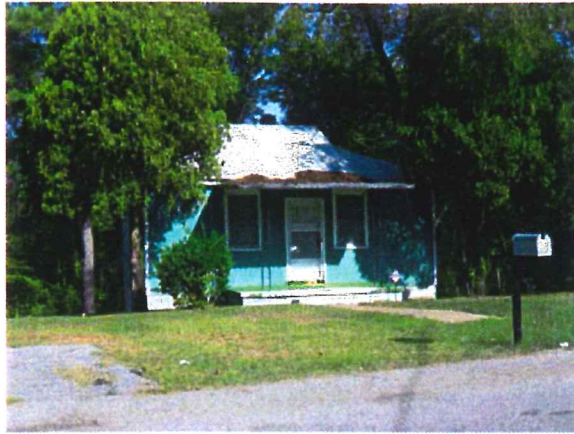
Substandard housing on Pineneedle Road in northern Hyatt Park
