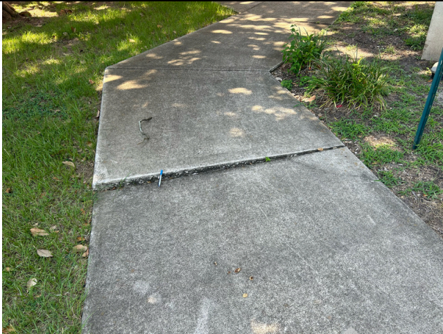
43. Site - sidewalk distress
