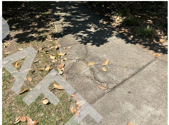
40. Site - sidewalk distress
