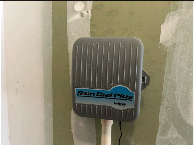
26. Site - irrigation controller
