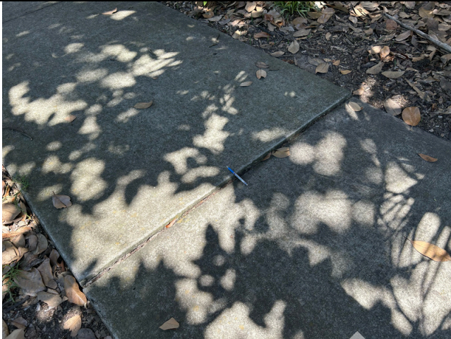
37. Site - sidewalk distress
