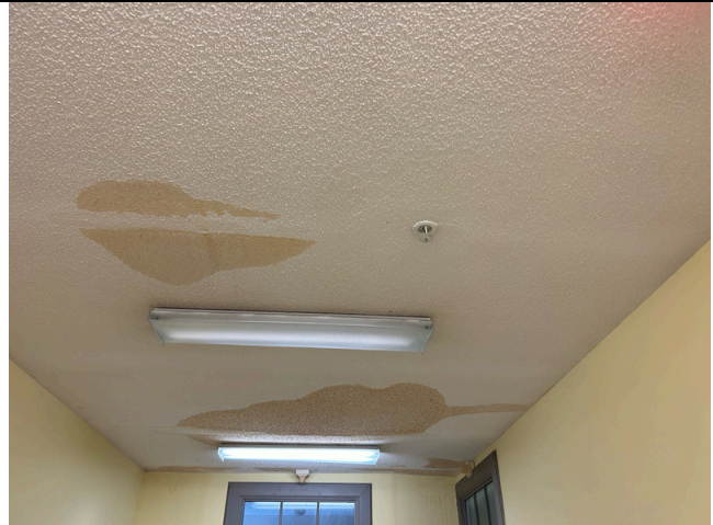
110. interiors - old plumbing leak / stained ceiling in corridor
