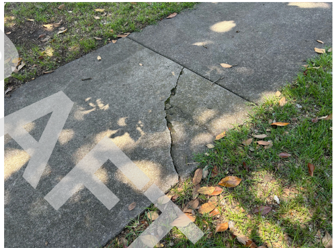
46. Site - sidewalk distress
