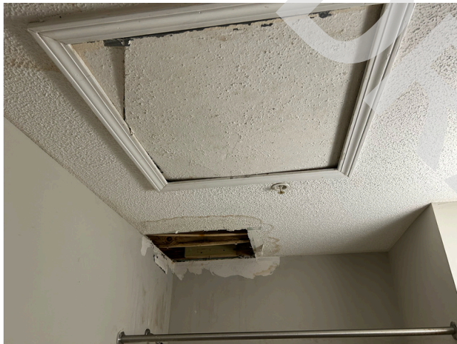
129. Interiors - unit 105 / old plumbing leak damage
