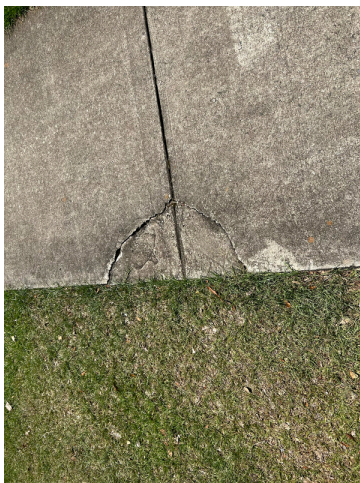
47. Site - sidewalk distress
