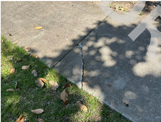
39. Site - sidewalk distress
