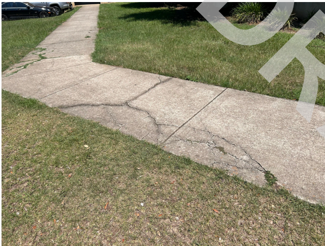
45. Site - sidewalk distress
