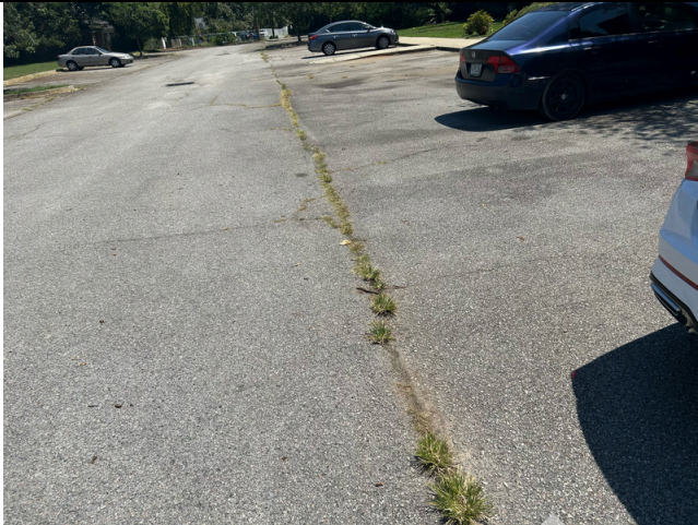
19. Site - asphalt at north parking lot (note vegetative growth)
