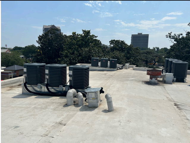
55. MEP - roof top HVAC condenser units
