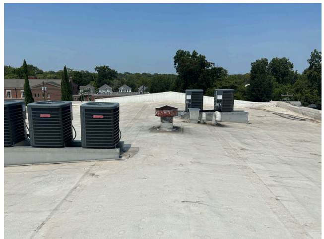
54. MEP - roof top HVAC condenser units
