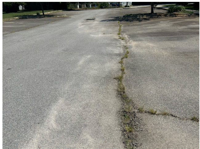
18. Site - asphalt at north parking lot (note vegetative growth)
