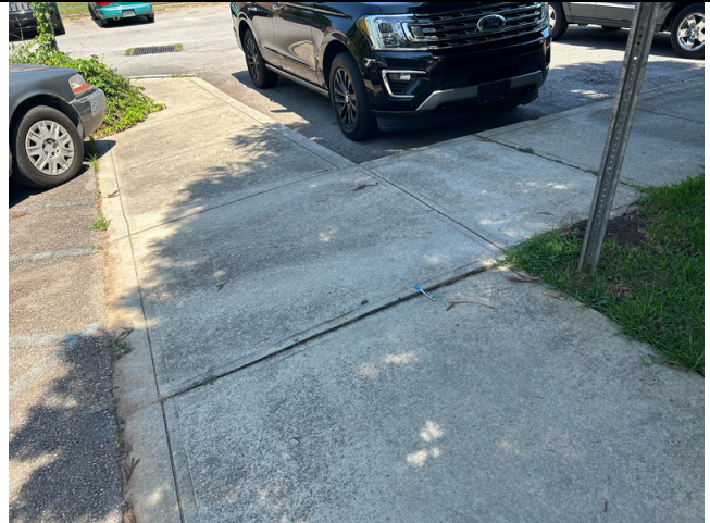
44. Site - sidewalk distress
