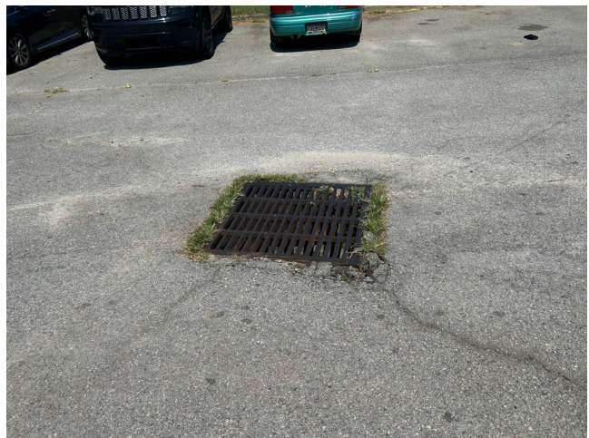
24. Site - area drain at drive lane (note vegetative growth)
