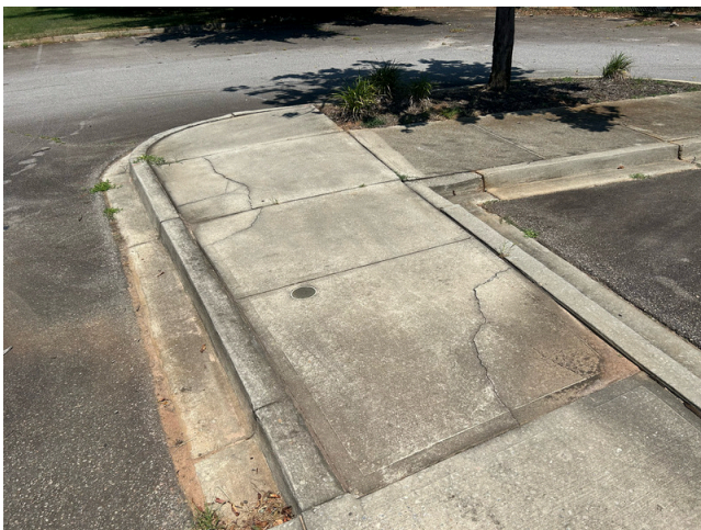
41. Site - sidewalk distress
