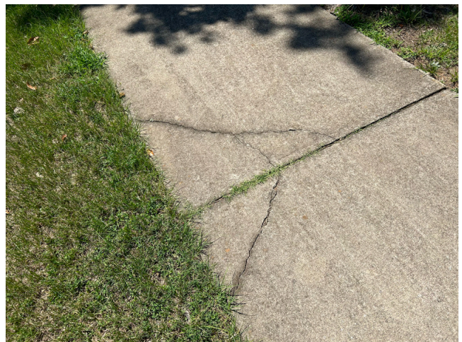
42. Site - sidewalk distress
