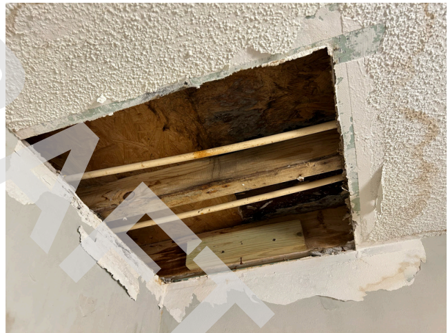
130. Interiors - unit 105 / old plumbing leak damage
