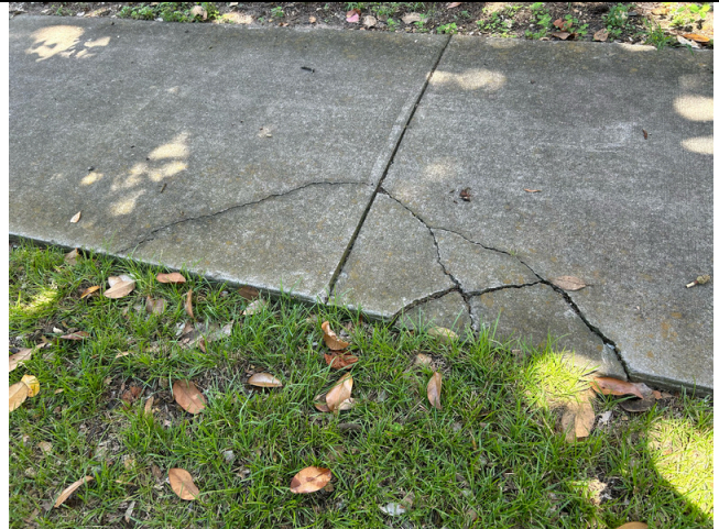
38. Site - sidewalk distress
