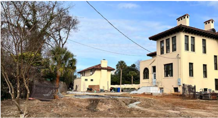
Site work has started for the D/DRC approved garage at 303 Saluda Avenue
