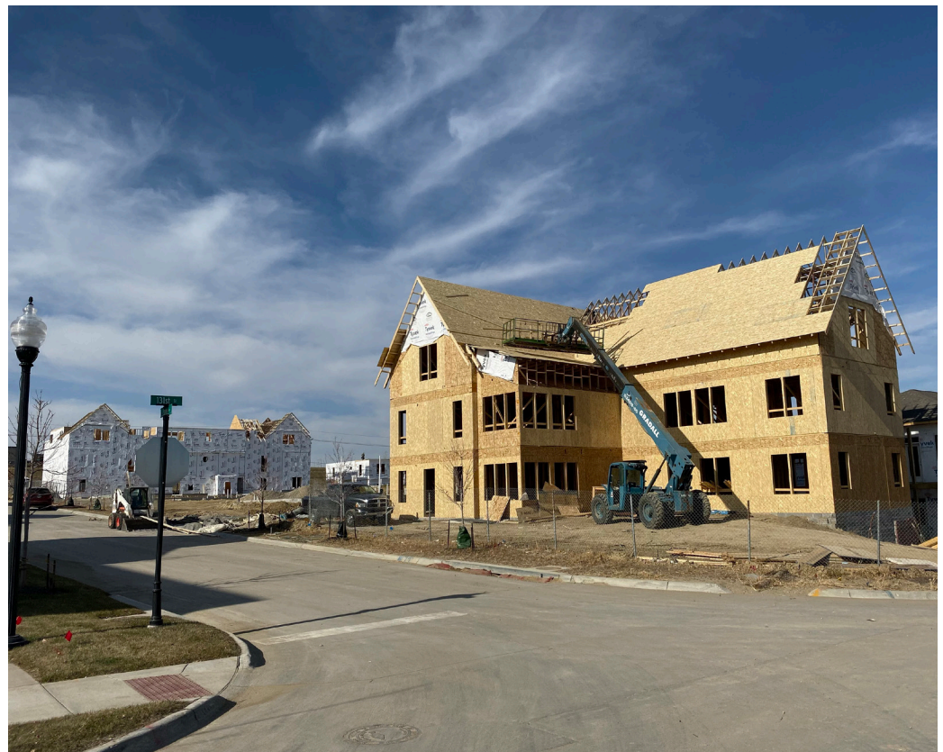
Figure 2.4 The simple forms, smaller size, and compatibility with Type V construction help maximize affordability and investment returns, and are consistent with the construction strategies familiar to most residential homebuilders, as shown in this under-construction MMH project in Papillion, Nebraska.
